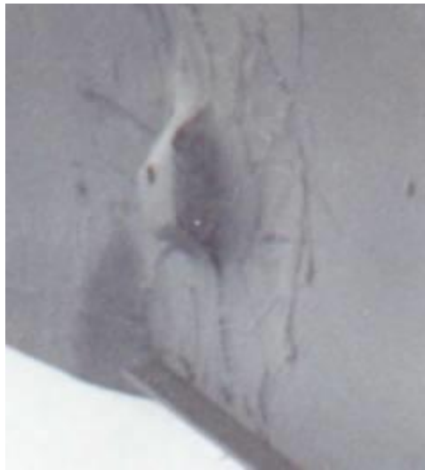
Figure 2. Upper side of undertray after fiberglass patching and painting.
